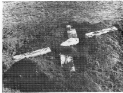
The base for The Georgia Guidestones® was set upon bed-rock and the giant "paddlewheel" is shown shortly after the concrete was poured.
