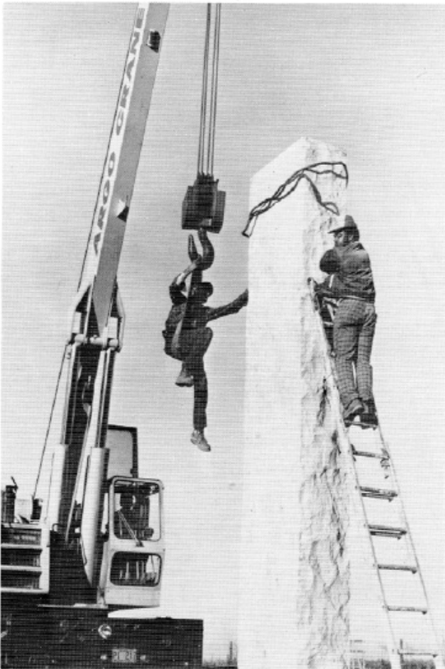
Workmen take cables loose as one of the Guidestones is placed in its rightful position. The rock-pitched finish on the sides is in accordance with "Mr. R.C. Christian's" instructions, that the finish conform as nearly as possible to the natural state of the granite as it is quarried.
