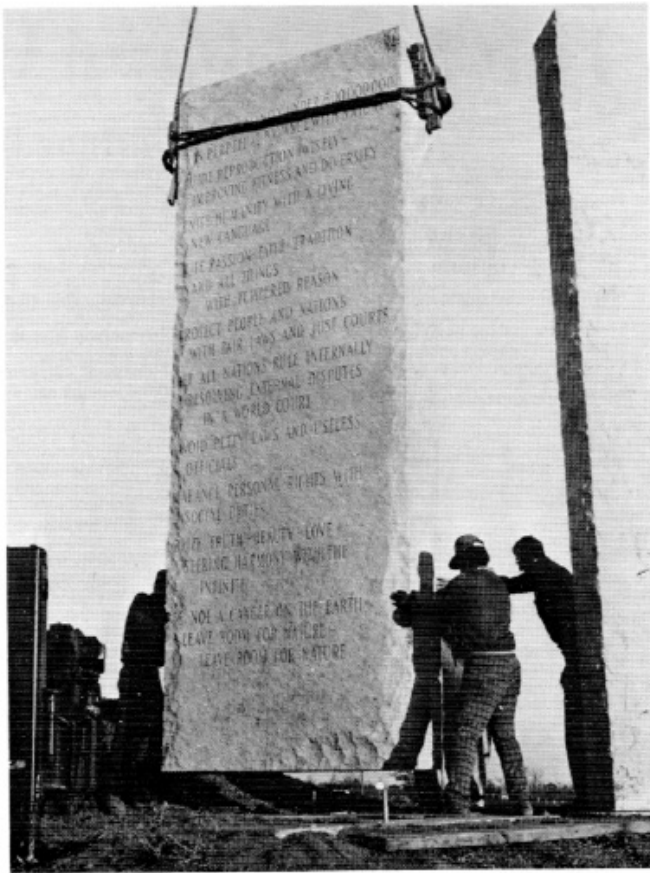
"Ever so gently!" describes how the crane and setting crew handled the stone sections and their enormous weight. As shown above, stainless steel dowel pins were placed in each of the granite bases and the upright sections were set on the pins.
